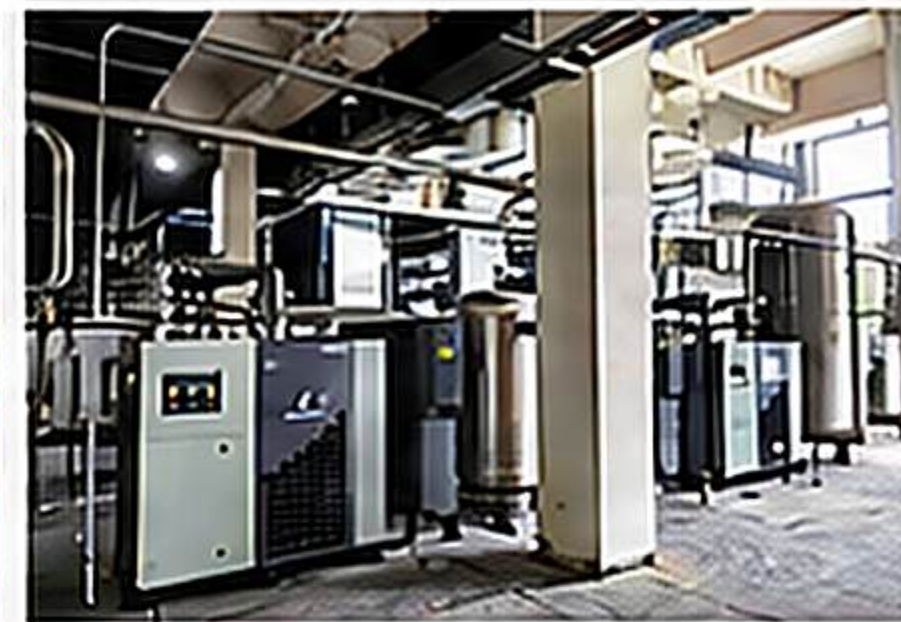
End User Pharmaceutical Co., Ltd. Equipment Refrigerated dryer 4 sets (28.5 m³/min per set)
