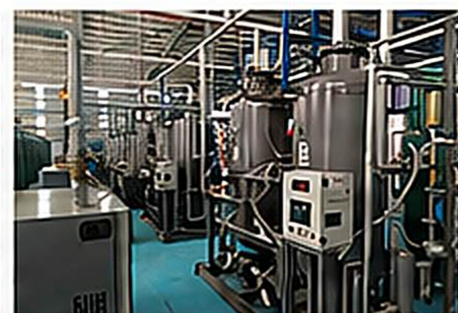
End User Automotive Equipment Refrigerated dryer 5 sets (3 m³/min per set)
