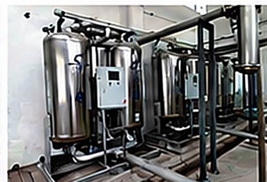
End User New Energy Industry Equipment Refrigerated dryer 8 sets (55 m³/min per set)
