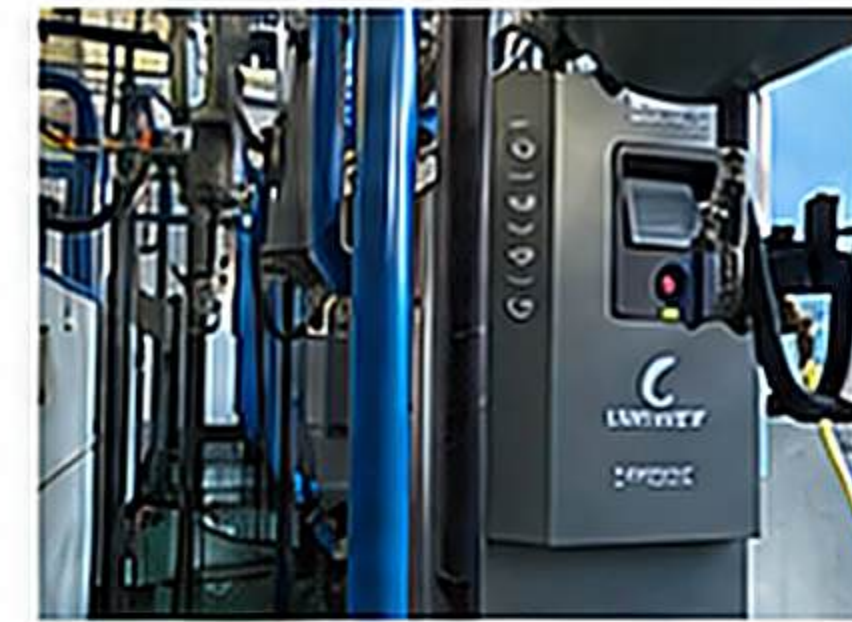
End User Extra-high Voltage Industry Equipment Refrigerated dryer 50 sets (50 m³/min per set)
